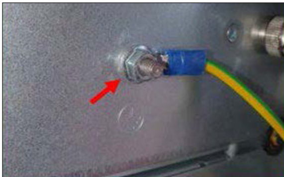
Figure 27 Ground Cable Disconnection
