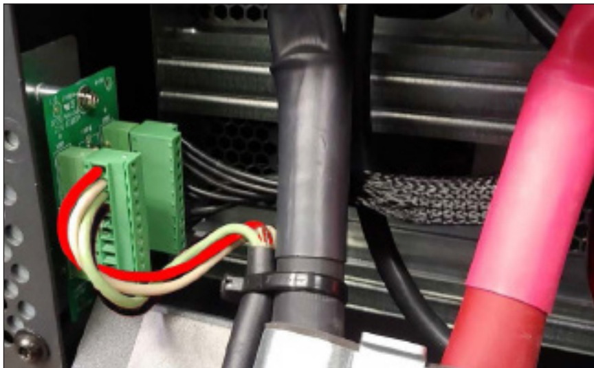
Figure 21 Battery Communication Wires Connected to the Screw Terminal
